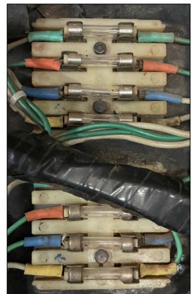
Fig. 4-3 Fuse holders and fuses
